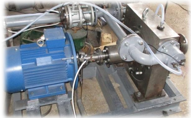
Figure 3 – Turbogenerator based on a vortex expansion machine with a strain-gauge coupling
